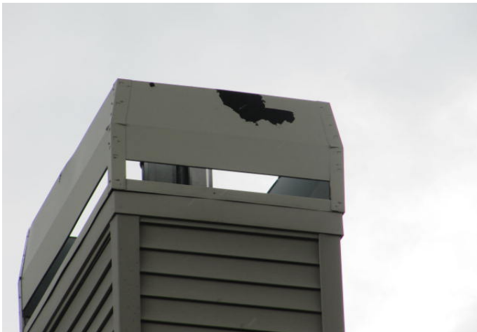
Chimney shroud with missing paint.
