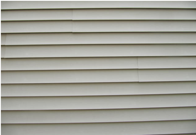
Typical siding condition.
