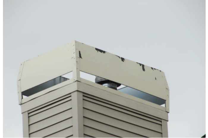
Chimney shroud with chipped paint.
